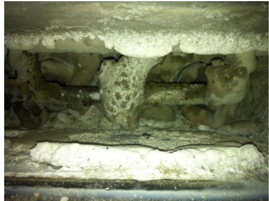
Heat exchanger fouling
