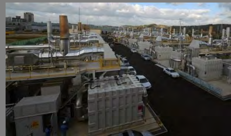
59MW fuel cell park
