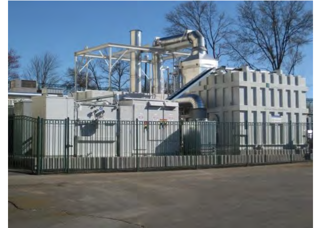
1.4 MW utility-owned power plant at CCSU – New Britain
