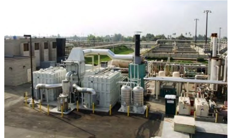
2.8 MW power plant at Inland Empire municipal water treatment facility Ontario, California
