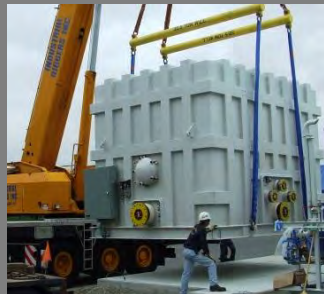
Completed module 1.4 megawatts
