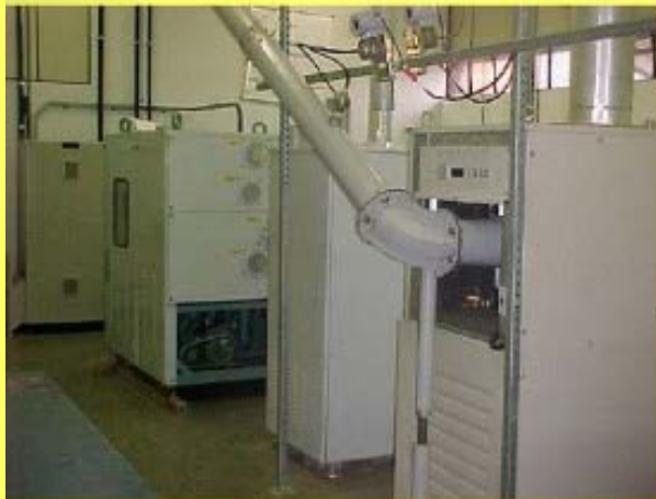
Microturbines and Chillers
