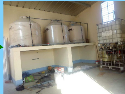
Storage Tanks Clearwell (Clean/Treated Water)
