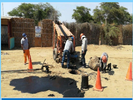
Sewage Back-Up Under Previous Conditions
