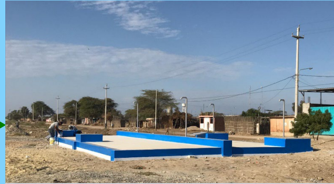
Ground Storage Tank (for Dry Weather Water Storage & for Water Particulate Settling/Clarification)
