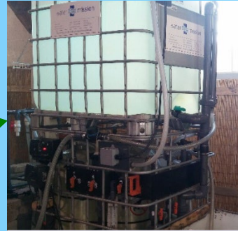
Water Mission's Living Water Treatment System (Filtration & Disinfection)
