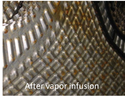
Heat exchanger plate
