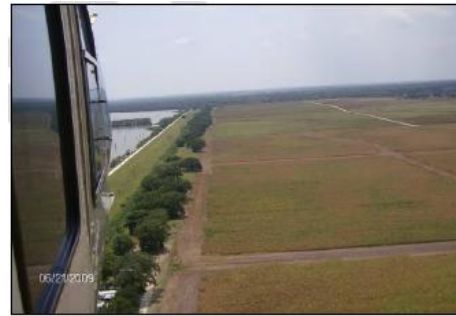
Figure 2-2. North Levee of Harris Reservoir with Prison Farm Land to the Right
