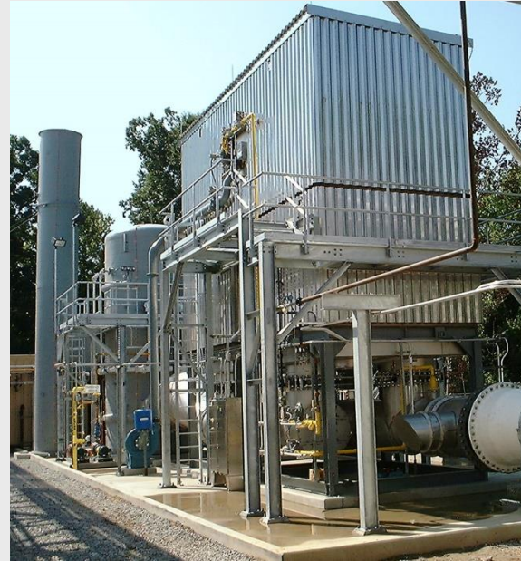
304L stainless steel shroud over an AL6XN reactor
