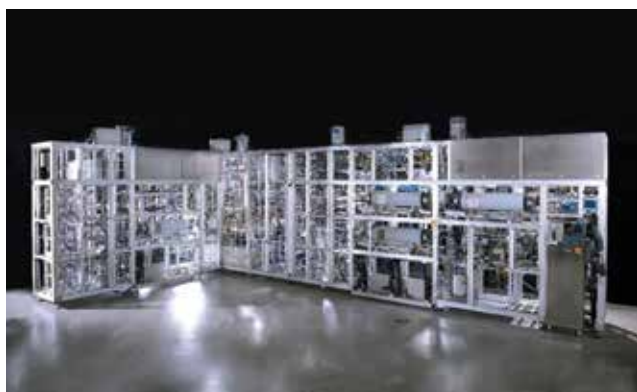
▲ Figure 1. Modular processes often have plug-and-play capability — i.e. , interchangeable process modules — like this pharmaceutical flow chemistry plant. Here, the modular design facilitates installation and reduces the process footprint.
