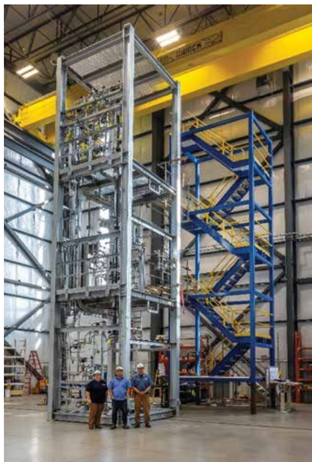
▲ Figure 3. Modular process units are often constructed offsite and reassembled or installed at the final facility location. Fabricating the unit on a modular skid reduces construction time and cost, as well as the potential risk to employees.
