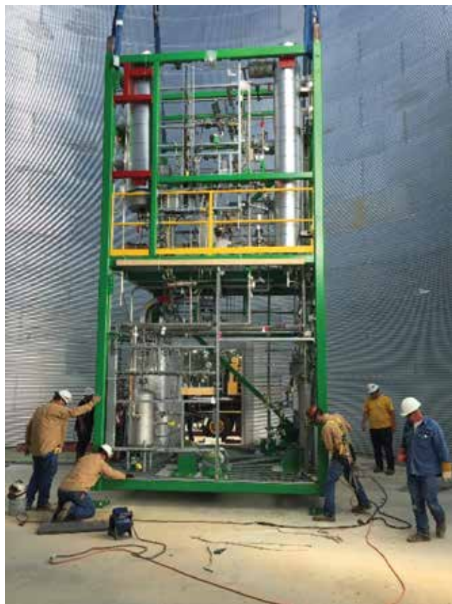
▲ Figure 4. Installing a prefabricated process module is often safer for workers than the more traditional route of stick-building a plant at the site.
