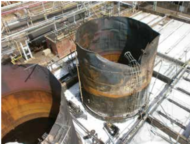
▲ Two storage tanks exploded after a lightning strike at a polymer plant in Bristol, PA (1).
