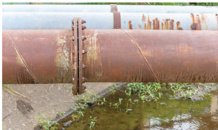
▲ A leak occurred in a process pipe years after it was shut down and “emptied.” It is likely that someone made a mistake during the clearing and flushing steps.
