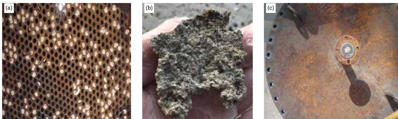
▲ Figure 5. A plant reboiler was experiencing much shorter run lengths than usual. Upon inspection, (a) the tube sheets were found to be plugged with (b) a polymer that had a different texture than previous polymers, which suggested the polymer was growing in a stagnant area. (c) The foulant also plugged the tower drain line.
