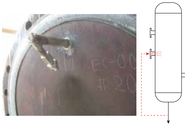
▲ Figure 12. Add a spray nozzle to reduce stagnant areas in external manways that are prone to clogging.
