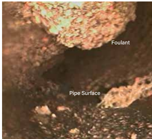
▲ Figure 6. A borescope is a useful tool for diagnosing fouling in long piping runs.
