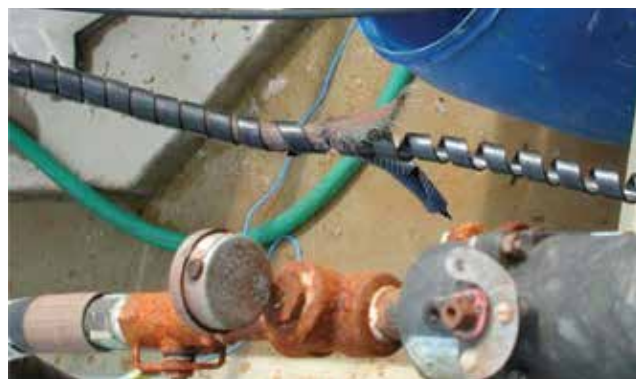
▲ Figure 4. A material verification program (MVP) is an important management system for reducing the potential for equipment failure. This hose failed because it was constructed of the wrong type of material. The hose failure caused the chlorine release incident described earlier. Source: (4).
