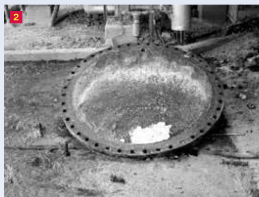
▲ Figure 2. Built-up pressure inside the tank caused the polymer catch tank cover to blow off.
