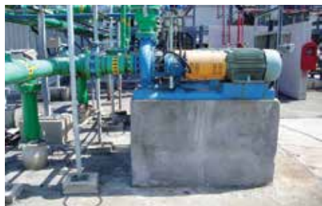
◀ Figure 4. A key monomer pump is elevated above the 500-yr flood elevation.
