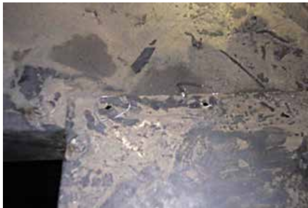
▲ Figure 19. Missing bolting hardware reduces the mechanical integrity of the tray, and is typically caused by vibration and/or loose installation.
