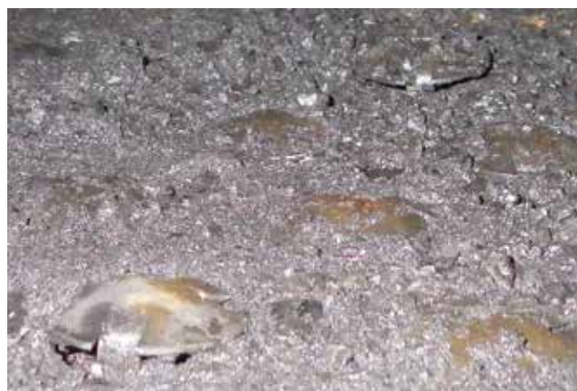
▲ Figure 10. Deposits above and below decks need to be removed to enable full movement of valves.
