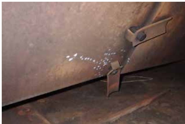
▲ Figure 16. This downcomer clip is bent from overtightening and has come loose, reducing the integrity of the attachment.
