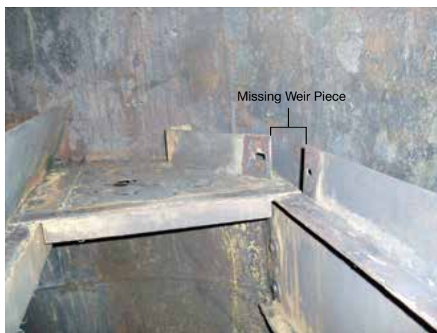
▲ Figure 18. The opening indicates the location of a missing piece of swept-back weir, which allows liquid to bypass the weir, causing maldistribution of liquid on the operating tray. The most probable causes for the missing piece are poor tightening of the bolting hardware or loosening of the hardware by vibration.
