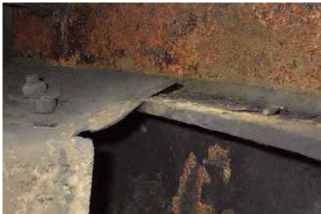
▲ Figure 20. Over tightening of ring clips can bend the perimeter edge of the tray deck.
