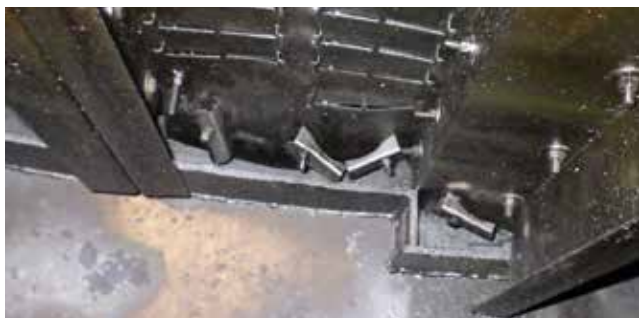
▲ Figure 22. A water explosion lifted this tray from its supports.
