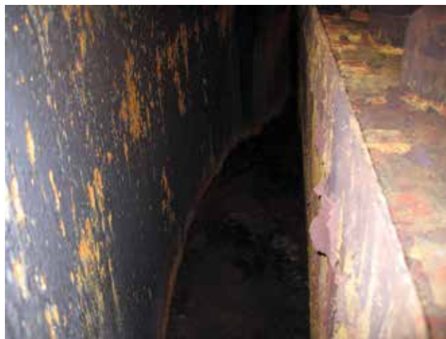
▲ Figure 7. Loose scale should be scraped or brushed off all surfaces to prevent flaking off into the process.
