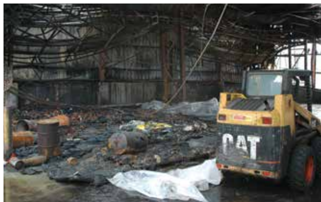
▲ Figure 5. Despite extensive damage to this storage facility, investigators were able to pinpoint the origin of the release because of witness statements.
