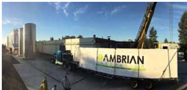
▲ The first EcoVolt Reactor was installed at Lagunitas Brewing Co. in Petaluma, CA.
