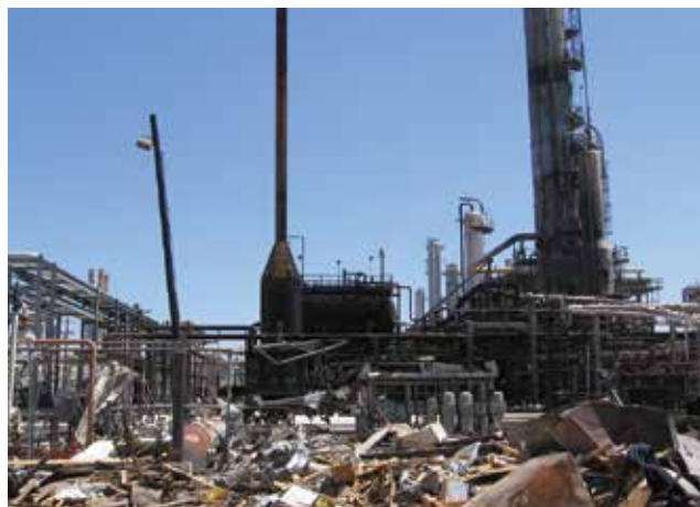
▲ Figure 3. The overflowing of a tower being started up set in motion a chain of events that led to a vapor cloud explosion and fire at the BP Texas City refinery. Source: U.S. Chemical Safety and Hazard Investigation Board.
