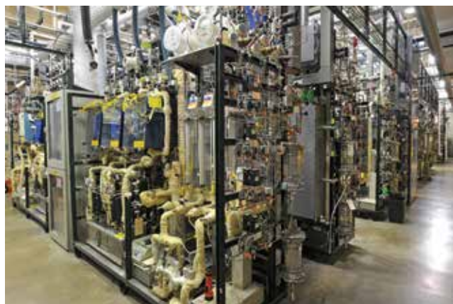
▲ Figure 1. Pilot plants come in a variety of sizes, but are typically smaller than process plants. This pilot plant, used for petrochemical research, is about average size.
