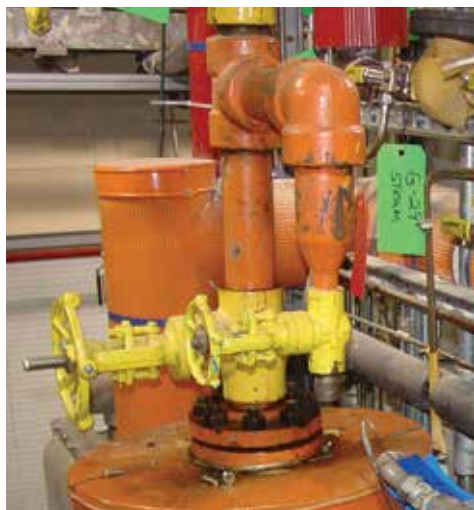
▲ Figure 3. Standard threaded piping and fittings are used on this pilot plant vessel.
