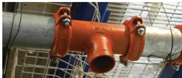
▲ Figure 11. Grooved piping and fittings are available in larger sizes, but these sizes are often too large for most pilot plants. Photo courtesy of Zeton, Inc.
