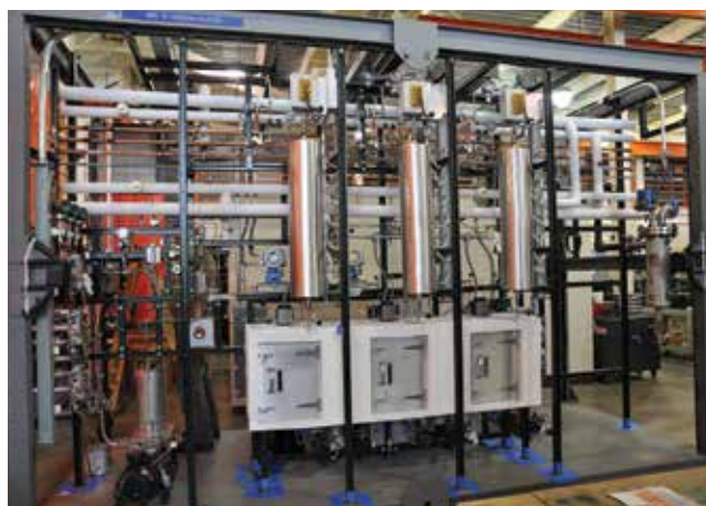
▲ Figure 15. This pilot plant has adequate room for maintenance and modifications.
