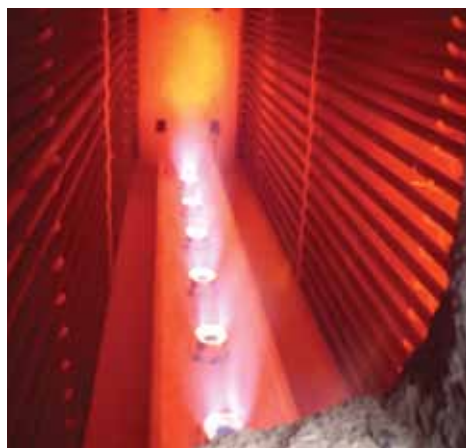
◀ Figure 2. Individual freestanding burners located in the middle of the firebox provide radiant heat for the tubes lining the firebox walls.
