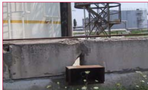
▲ June – A hole in the wall of a tank farm containment dike
