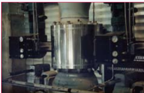
▲ April – Insulating cover on a long-bolt flangeless valve
