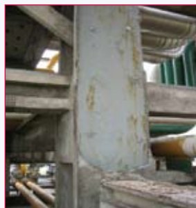
▲ May – Damaged fireproofing on a pipe bridge support column
