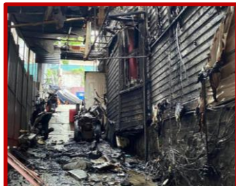
Figure 1: Damage to buildings caused by a lithium-ion battery fire.
