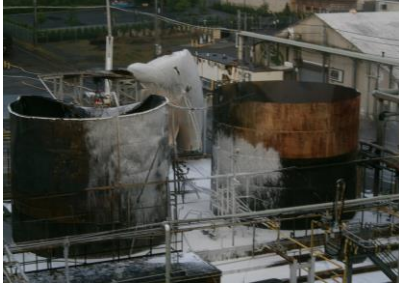
Figure 2. Tanks after the fire
