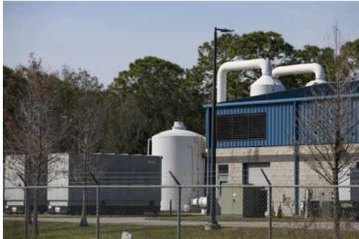
Rajah 1. Loji rawatan air Oldsmar, Florida
