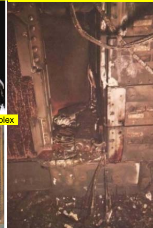
Section of CM interior after fire
