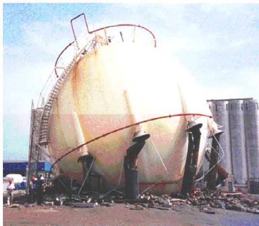
Corrosion Attacks Structural Supports
