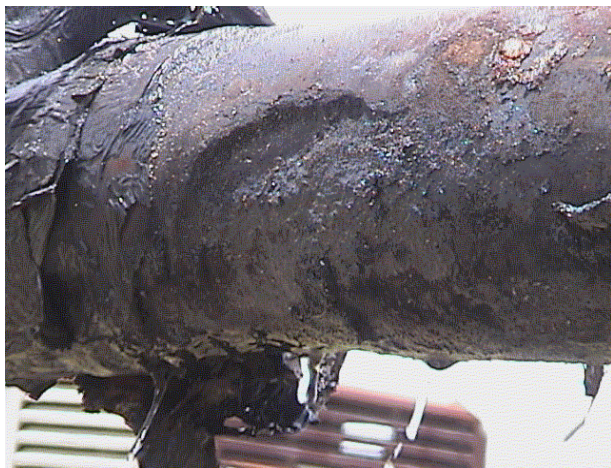
Corrosion Attacks Piping
