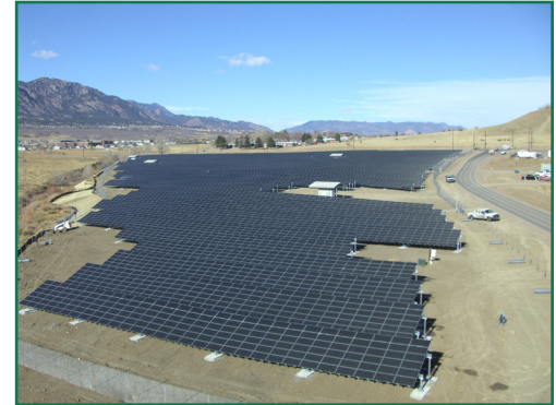
Solar photovoltaic (PV) facility at a former landfill in Fort Carson, CO.
